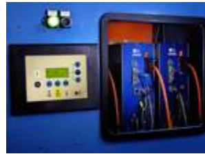
RFID on an Industrial PLC
