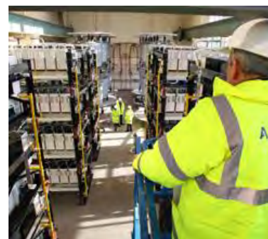
Alstom Grid UK HDVC Power Systems
